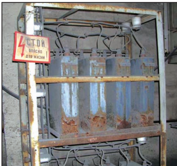
● Photo 2.3.2.2 Exploited PCB-containing capacitors with corroded cases.
