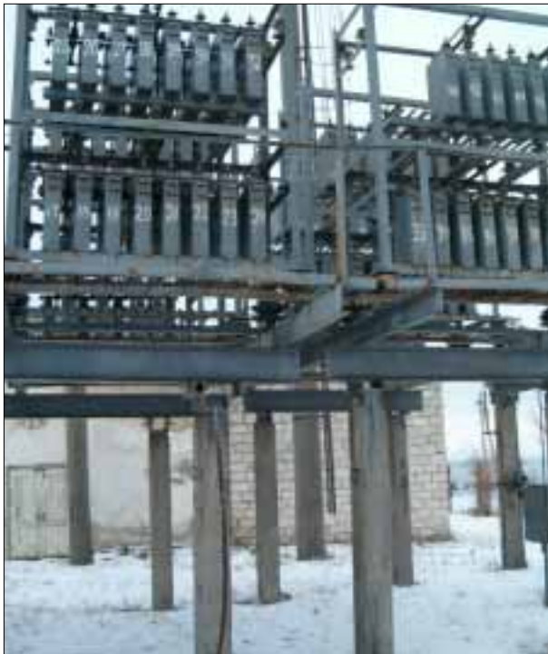
▲ Safe storage of capacitors will prevent releases.
