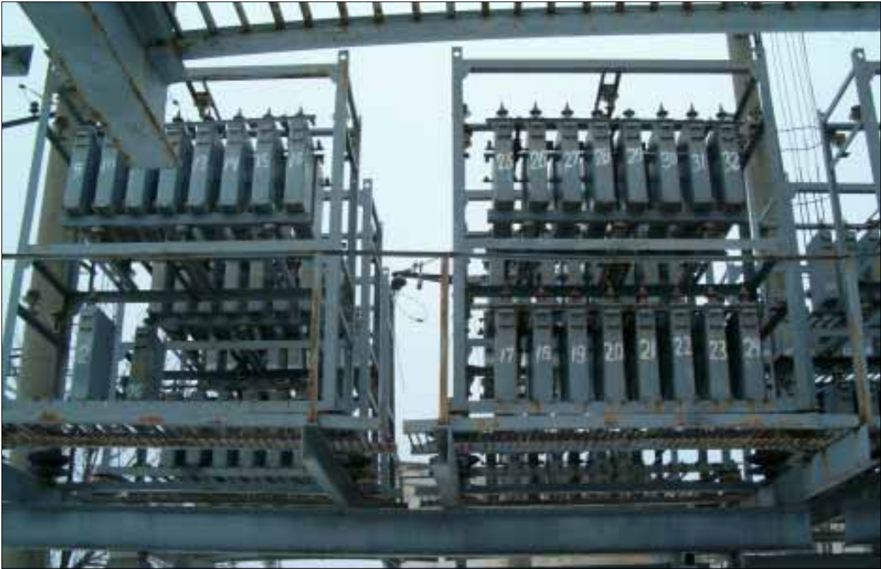
▲ Block of capacitors
