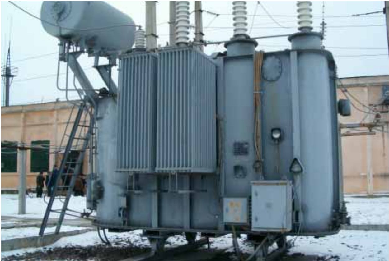
▲ Power transformer in operation "Moldelectrica", Orhei
