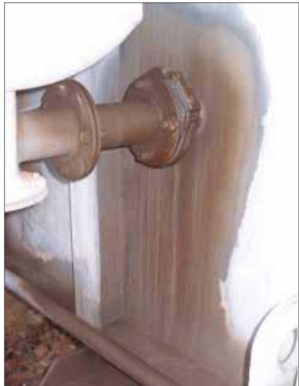
▲ Leakages of oil from the transformer
