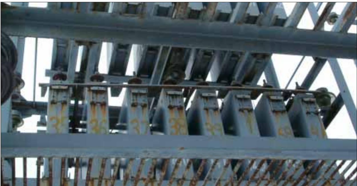
▲ Capacitor batteries in blocks
