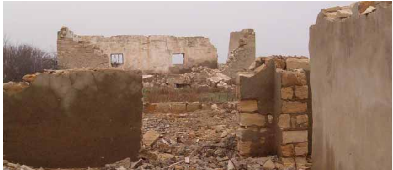
▲ Destroyed warehouse: looking for low cost solutions.
