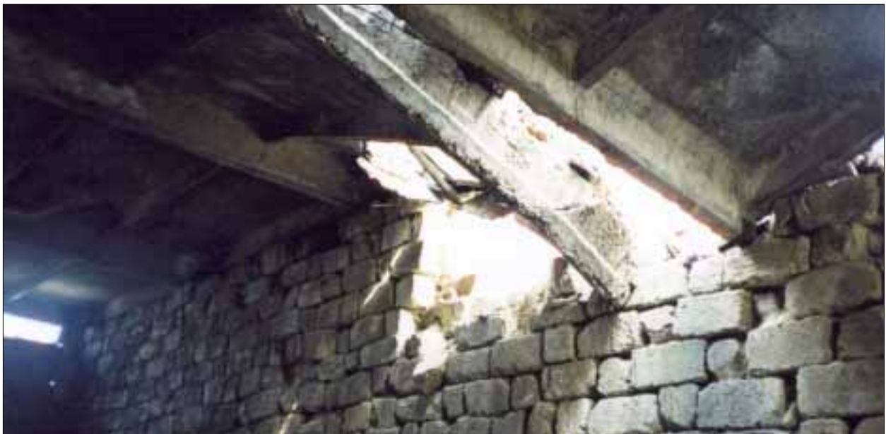
▲ The roof of the pesticides warehouse need to be repaired.
