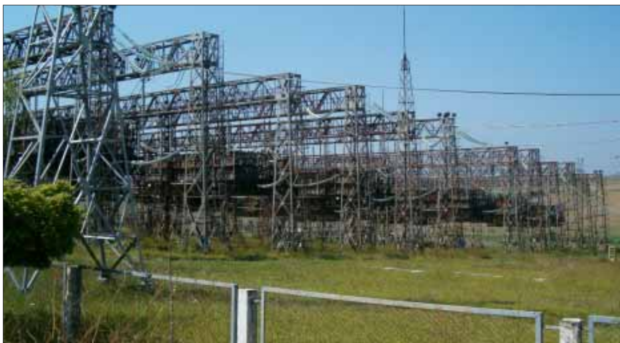
▲ Old capacitors at Vulcanesti station require urgent remediation measures.
